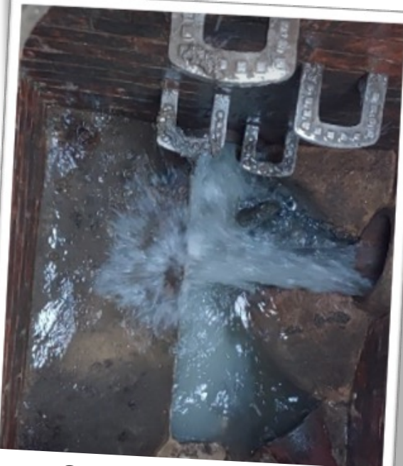
Gurnard, Isle of Wight Large surface water misconnection
